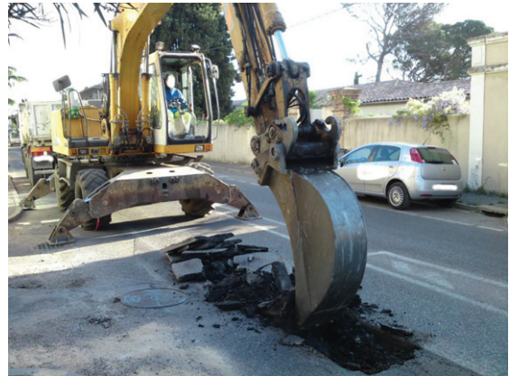
Fig. 3. Worker driving a pneumatic shovel and digging a trench on a road.
