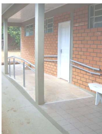
Figure 2: Access to classroom by ramp, with handrails at two heights on both sides. (ANDRADE, 2010)
