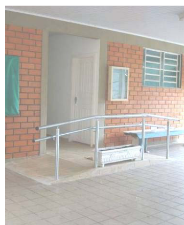
Figure 3: Ramp created to allow access in all public spaces, like secretary, teachers room, labs, library and toilets. (ANDRADE, 2010)
