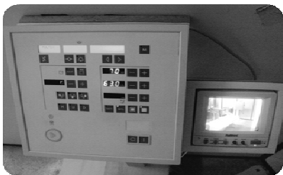
Figure 5: Control panel with display.
