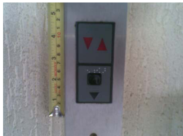
Pic. 5 - Button panel of the elevator installed upside down, jeopardizing the Braille reading. Source: Collection of photographic project ERGO-POLIS/GREPE/UFRN
