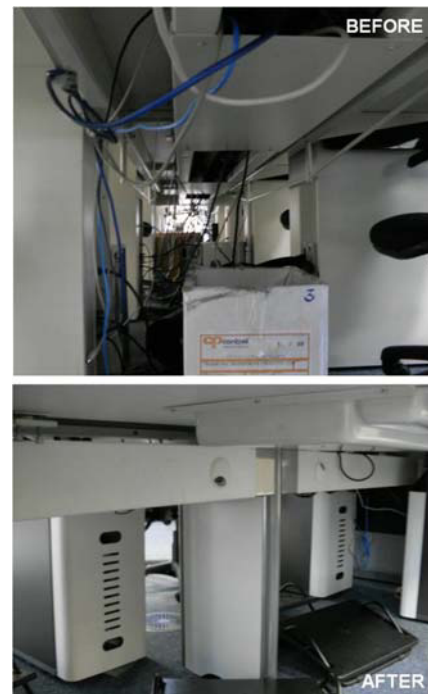
Fig. 6: Cabling, before and after
