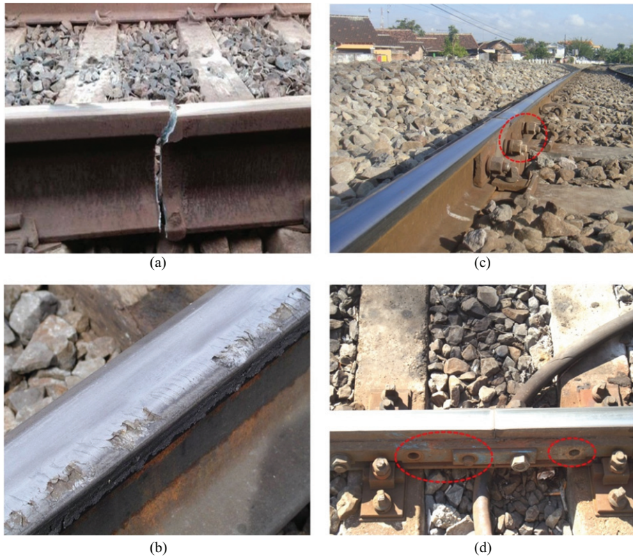
Fig. 1. Examples of track abnormalities (a) deformation with crack, (b) rusty deformation on rail top, (c) loose bolts, and (d) missing bolt.
