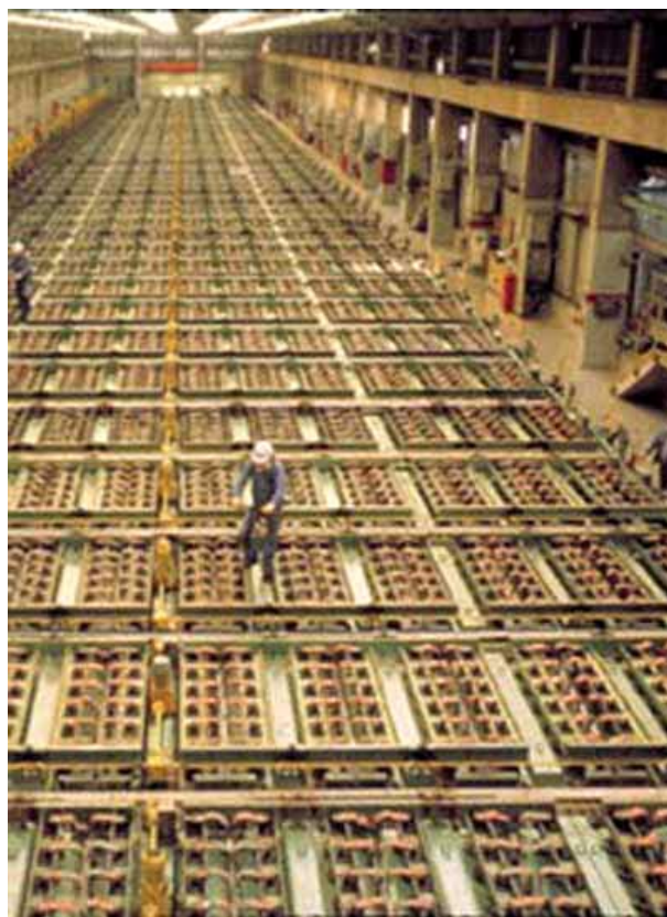
Although chlor-alkali plants are only responsible for 5% of mercury emissions in the atmosphere, chlorine producers in Western Europe have agreed not to build any new mercury processing plants, and many are looking at economically viable alternatives in order to comply with a total phase out of the mercury process by 2010 Courtesy: SPG Media
