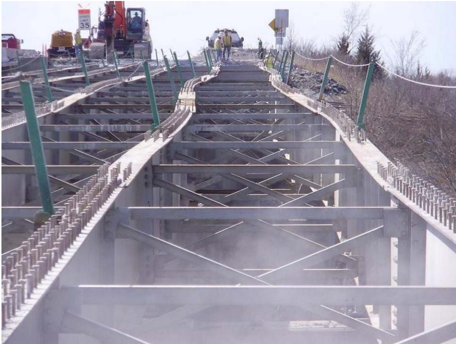
Fig. 17. Lateral buckling of girders following deck removal in Missouri, USA [28].
